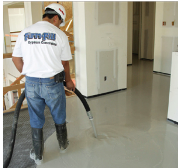
Firm-Fill 3310 poured gypsum concrete underlayment and Sound Mat II recycled rubber pad add strength and sustainability to the 2009 New American Home in Las Vegas.
