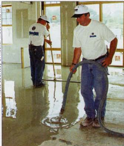
Gypsum concrete floor underlayments are installed over wood or concrete surfaces to achieve a sound-rated, fire resistant surface for floor coverings.
