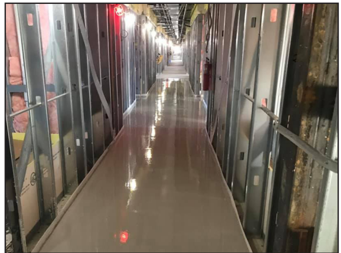
Finished pour of Firm-Fill® CMD in hallway - the gypsum dried enough to walk in within 90 minutes
