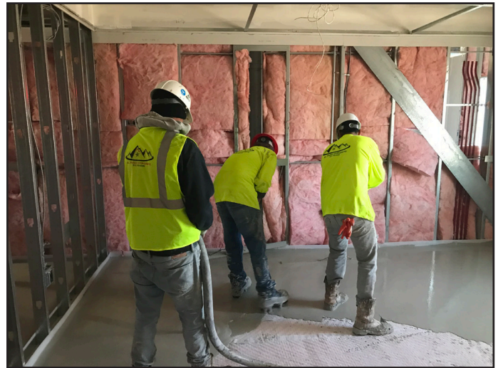
The second lift of Firm-Fill® CMD is installed over Firm-Fill® SCM-250 at 1" in depth
